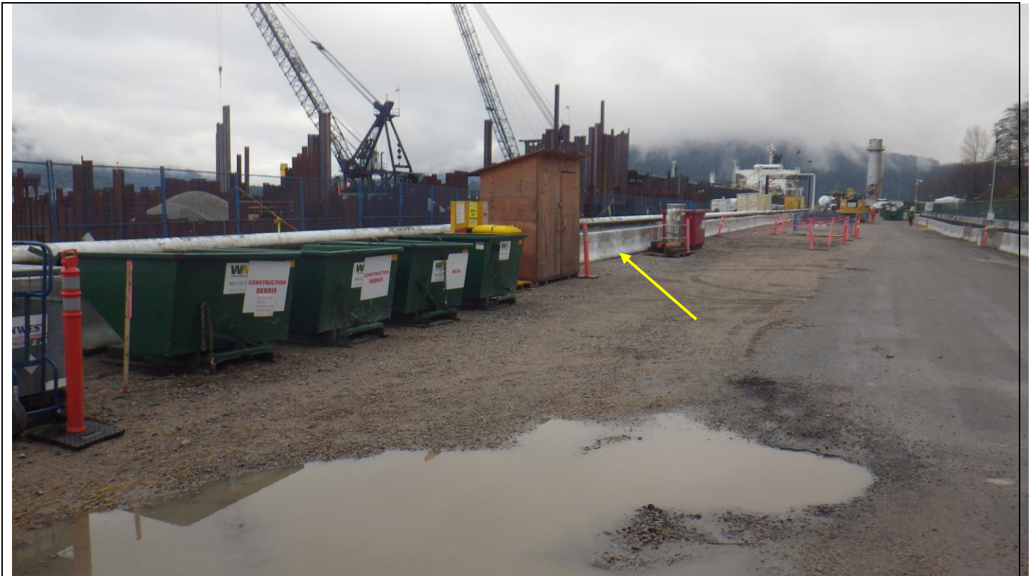
Photo 5. White concrete lock blocks (yellow arrow) placed along shoreline to avoid runoff into the marine environment from the area where concrete column mixing will occur.
