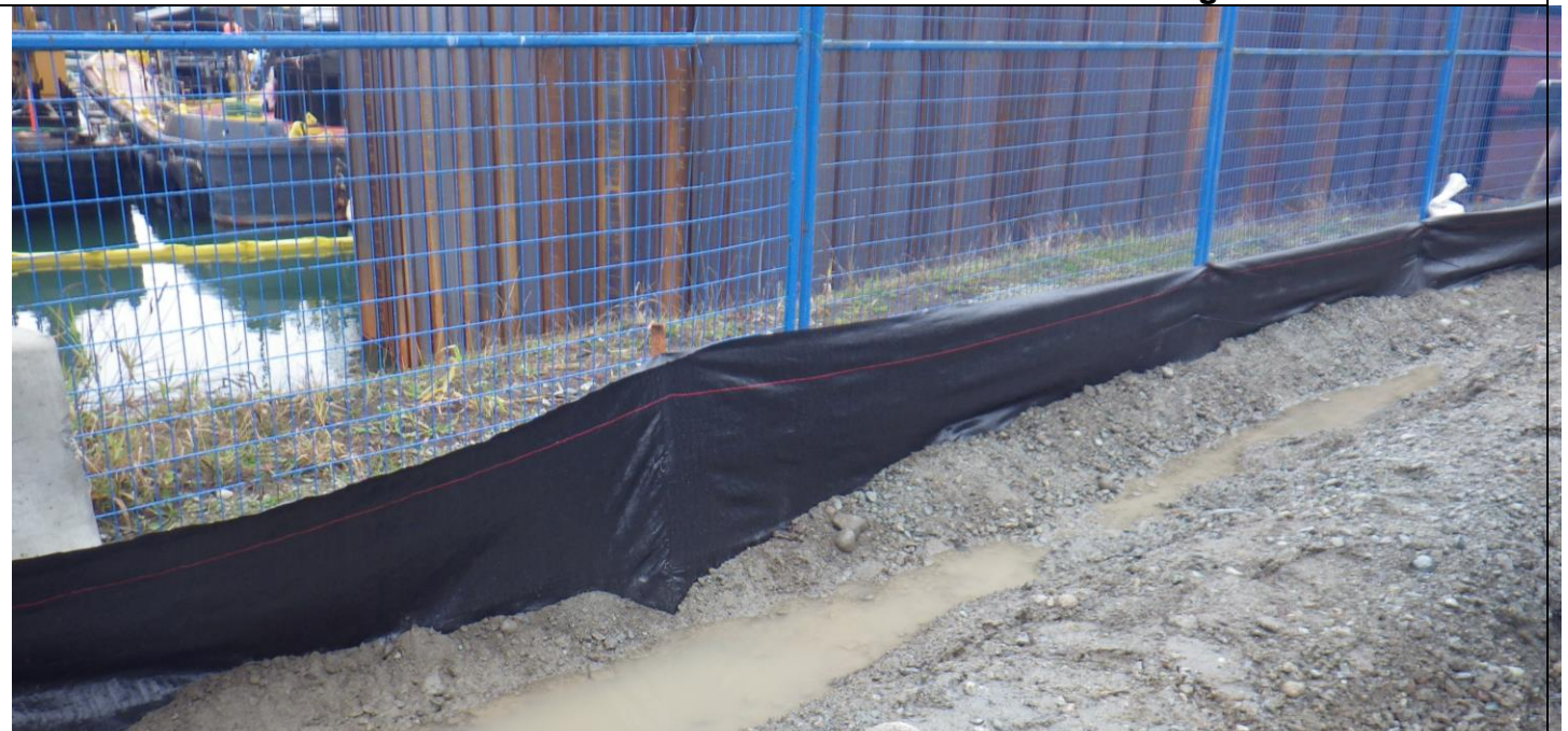
Photo 6. Berm and sediment fence installed as additional measures to avoid runoff into the marine environment from the area where concrete column mixing will occur.
