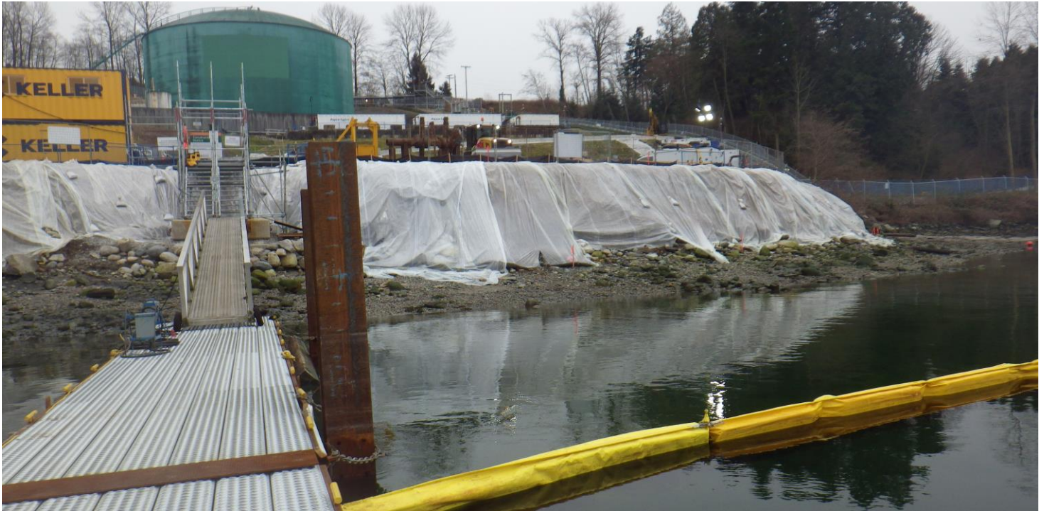
Photo 1. Polysheeting along shoreline to reduce erosion; yellow turbidity curtain in place to contain turbid water.
