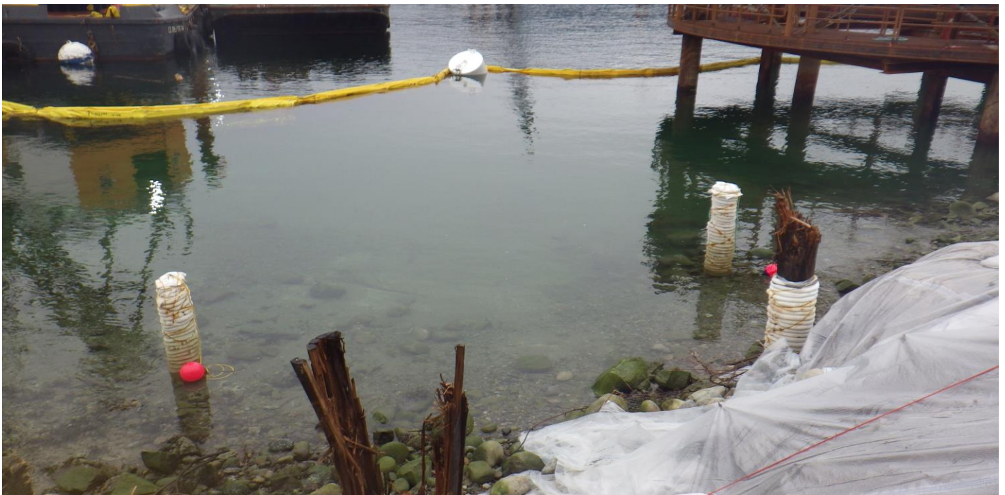
Photo 2. White sorbent rings placed around creosote piles remaining from demolition of small utility dock. Piles to be removed at a later date.
