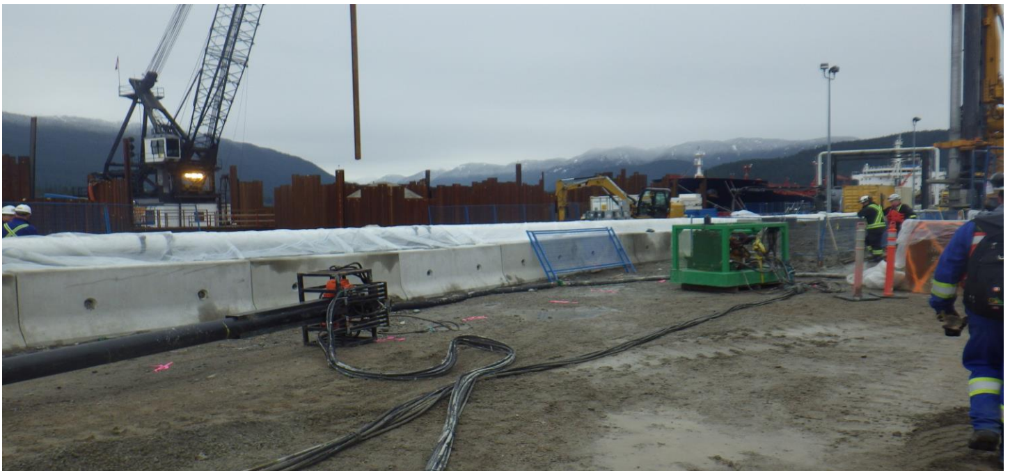
Photo 4. Lock blocks in place to prevent erosion of sediment-laden water or other materials into the marine environment from on shore works.
