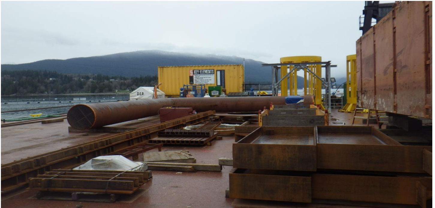
Photo 5. Base of the new bubble curtain that will be placed on the seafloor to further attenuate underwater noise at depth during impact pile driving. The new curtain will consist of two ‘L-shaped’ sections that join together to form a square.
