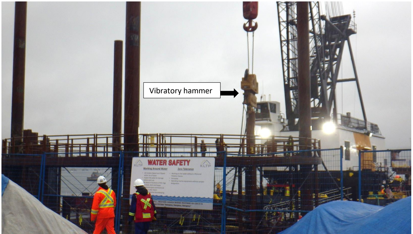
Photo 3. Installation of the template at sheet pile cell 8 by vibratory pile driving.
